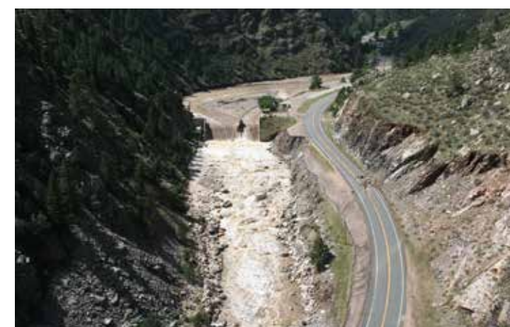
Idylwilde Dam pre- (middle) and post- (bottom) 2013 flood. Sources: Loveland Water and Power, CDOT
